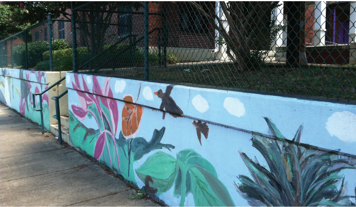
Mural painted on the retaining walls surrounding Southtown Court - Though many are in good condition, a number of the retaining walls at Southtown Court show significant signs of deterioration
